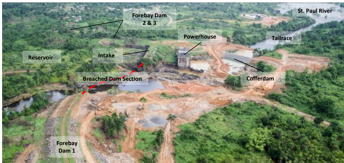
Figure 1 - Breached dam section with Intake and Mt Coffee Powerhouse in May 2014 (source: Airmed Liberia)
