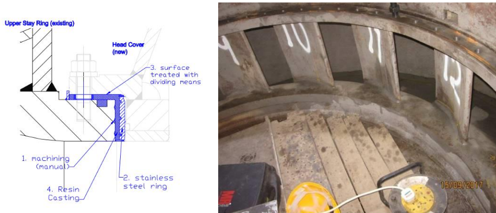
Fig. 5. Left: Sketch of modification of stay ring by insert ring and resin casting; Right: Method under implementation
