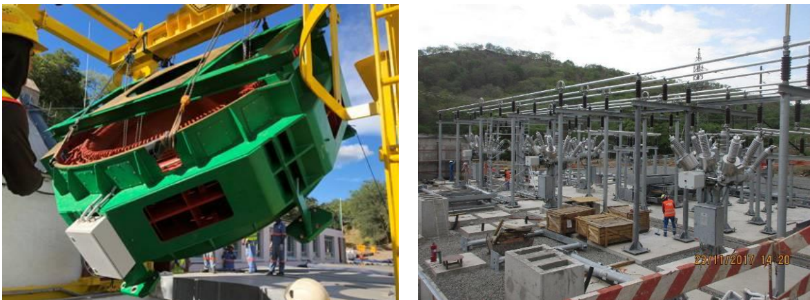
Fig. 3. Left: Lowering of the pre-assembled vacuum impregnation generator stator; Right: 66kV hybrid switchgears
