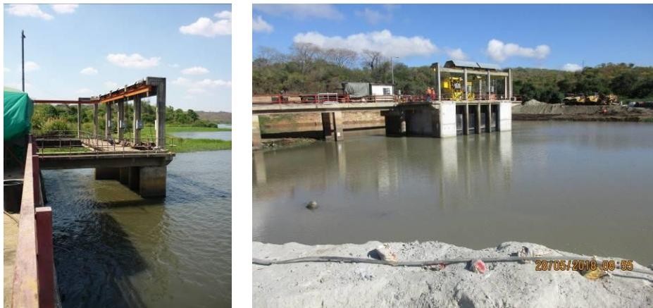
Fig. 2. Left: Nkula A intake structure before rehabilitation; Right: Nkula A intake structure after modification works
