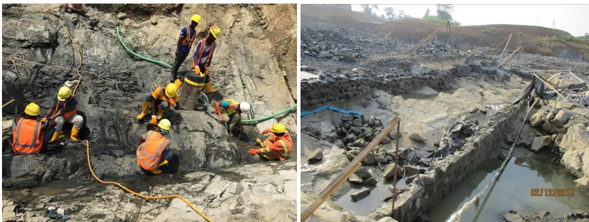
Figure 4 - Left: Foundation preparation using industrial type vacuum cleaners, Right: Walling off the section to be poured with mortar layer
