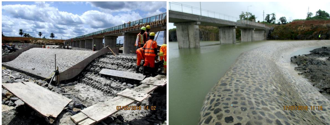
Figure 5 - Left: Use of shutter ply profiles and fish line for Final Shape, Right: Smooth finish of ogee spillway shape
